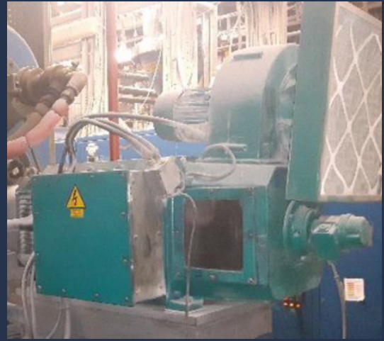
Figure 3 - DC motor with cooling fan
